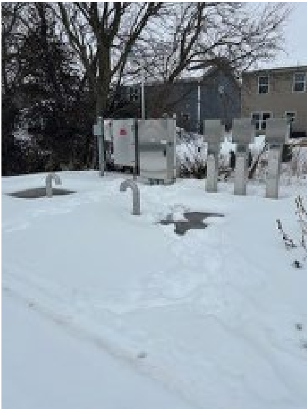
Newly added Sutter Place lift stations
