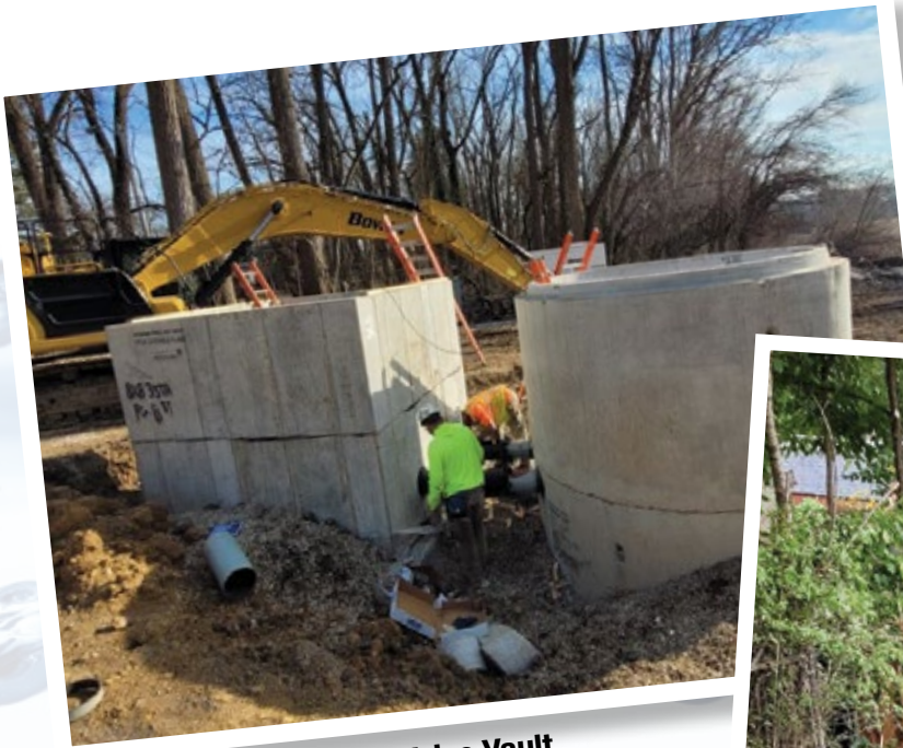
35th Street Wet Well & Valve Vault
