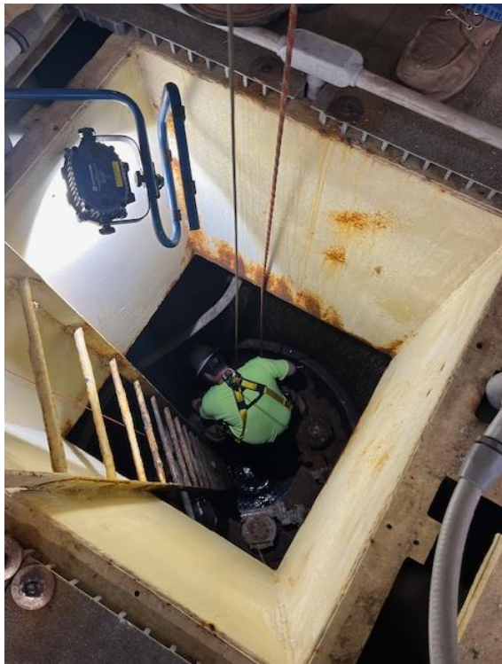
Backwash equipment at plant 2
